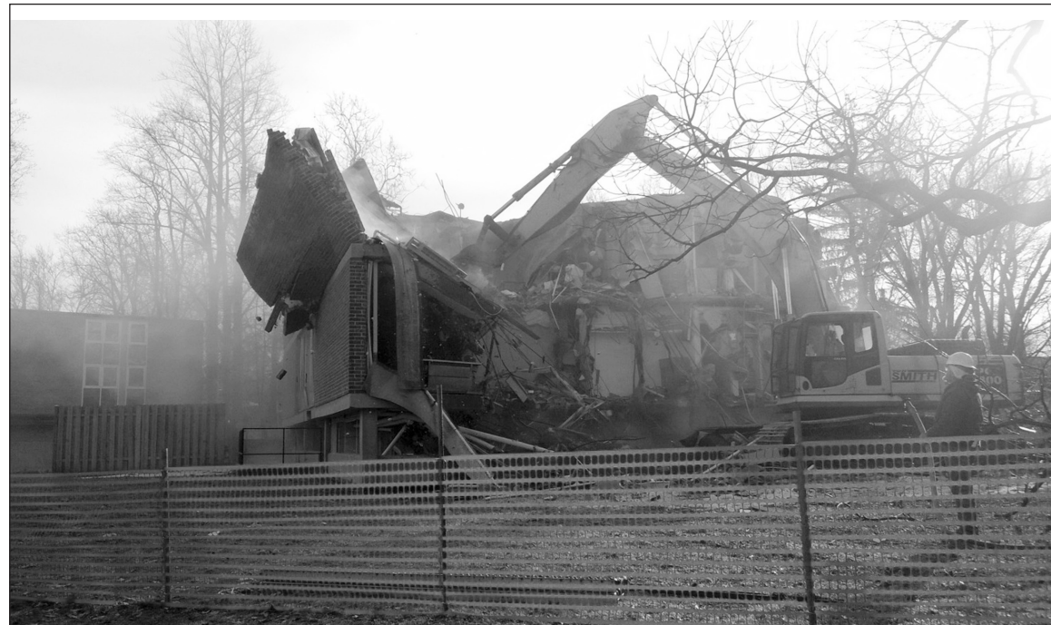
Demolition of former dormitory Mills Hall. The dorm was built in 1959. Photo by Richard Hauck '17
